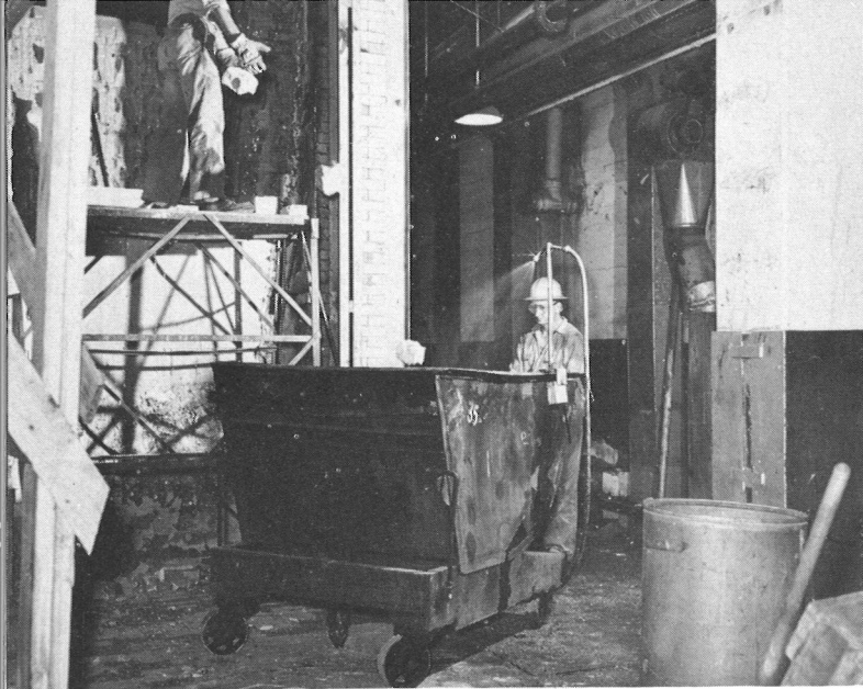
Furnace port bricks, also wet down earlier, are sprayed in rubble cart. Frank Guran tosses, Bernie Doran watches.
