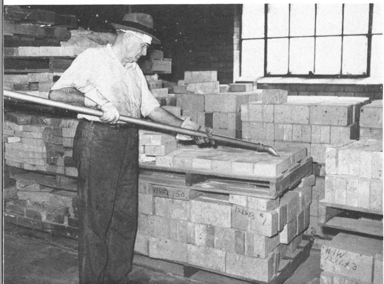
New bricks are vacuumed layer by layer as used. Dust control's thoroughness assures safety without respirators.
